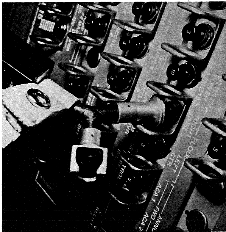
Reach Aid Closing Circuit Breaker
